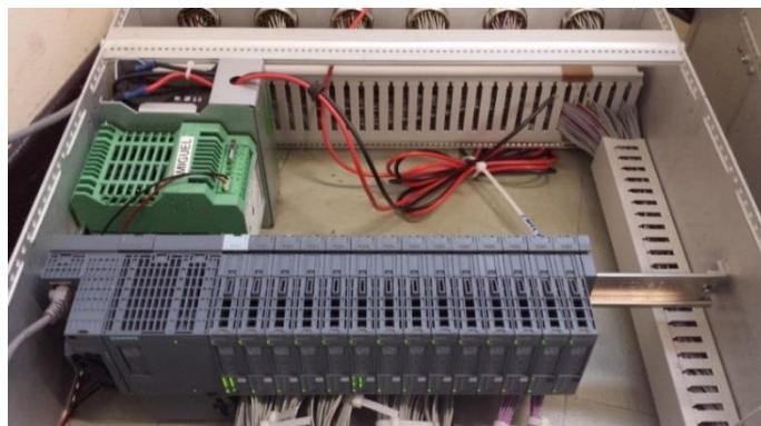
Figura 62. Rack de PLC.
